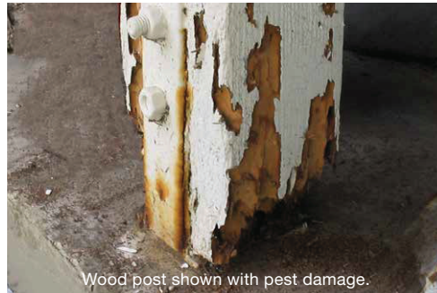
Wood post shown with pest damage.
